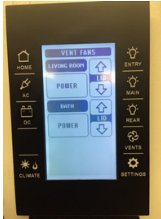
Figure VIII Remote Vent Fan Operating System
