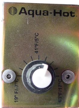
Aqua-Hot thermostat located next to water pump in water service bay
