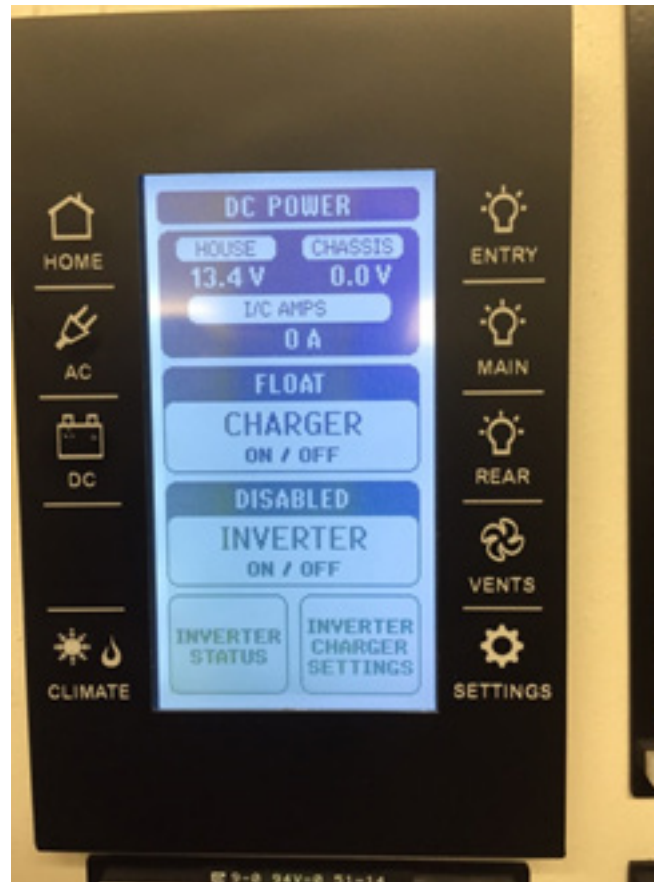
Figure III Direct Current Components and Status
